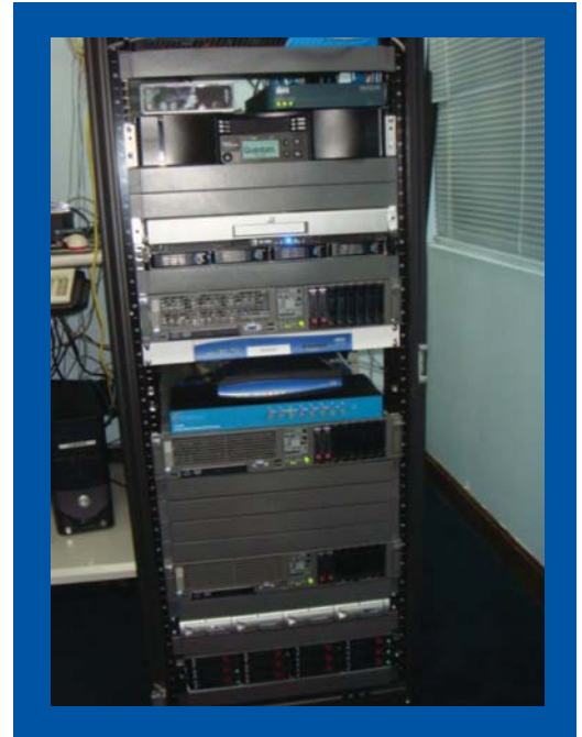
Server Room at MFIC. (This rack replaced an entire File Room!)
